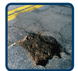
POTHoles/ DAMAGED PAVEMENT
